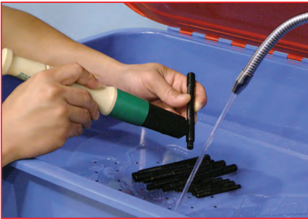
2. All hardware (and caps) should be cleaned and inspected prior to installation, looking for any shipping damage or defects.
